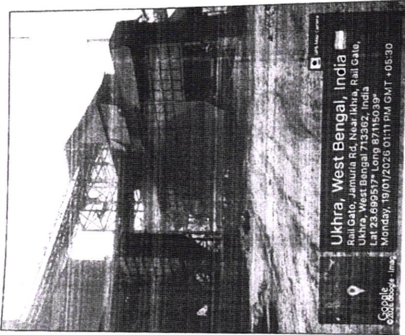
Stack of one no Bag filter at Cooler discharge of older 2x100 TPD Kilns missing (Pic 19)
