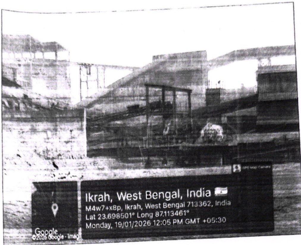
Broken conveyor canopies at Old DRI section (Pic 15)
